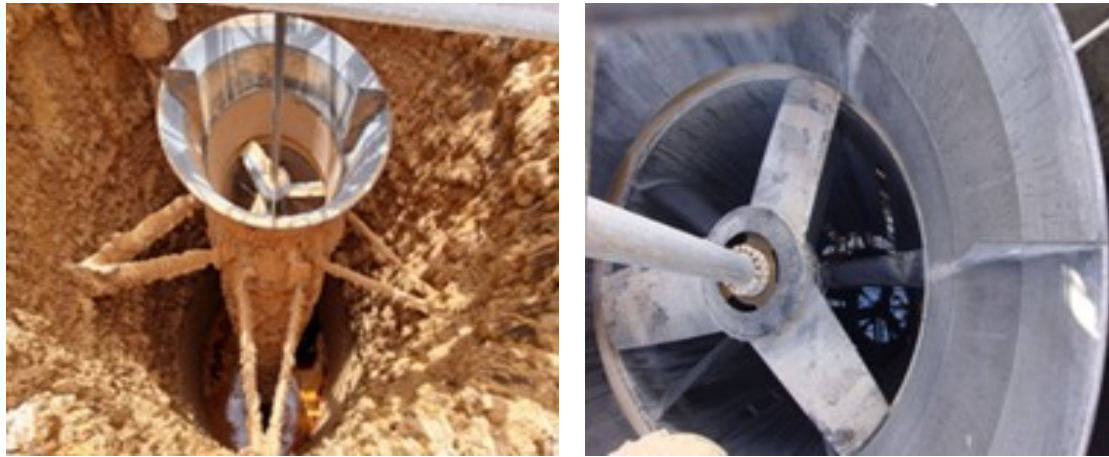
Figure 2. Tank draft tube. Left: Tank online for 175 days (vs expected residual life 230 days), Right: Clean draft tube.
